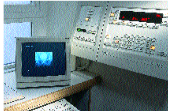
Fig. 4. Control room showing the generator control desk. The GCF controls are on the left.
